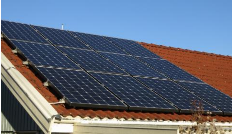
20 sqm solar panels on garage roof, Nov 2012 Generated 2700 W at noon March 10, 2013
